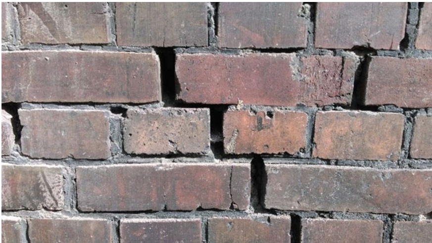
Fig. 6 Fragment of the external wall with damaged vertical and horizontal joints
