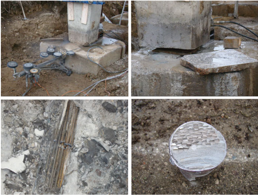
Fig. 7 Progressive damage of column and tendons on bridge S101 [23]
